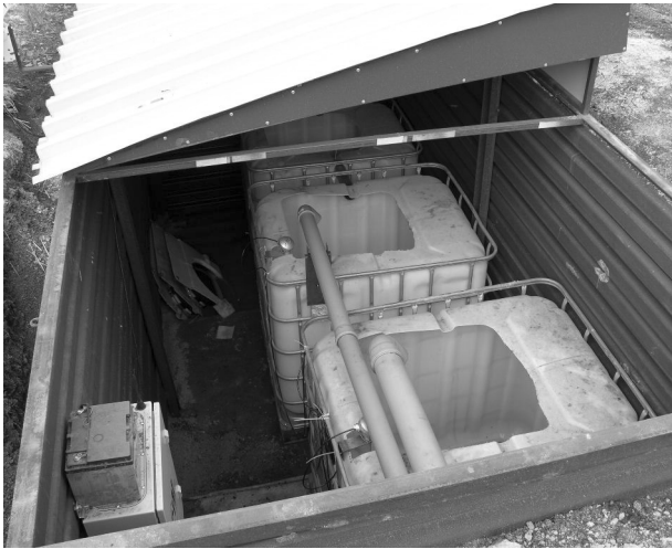
Fig. 1. The collector is piped into the 3 tanks imbedded in sheet metal panelling pits separately for each variant
