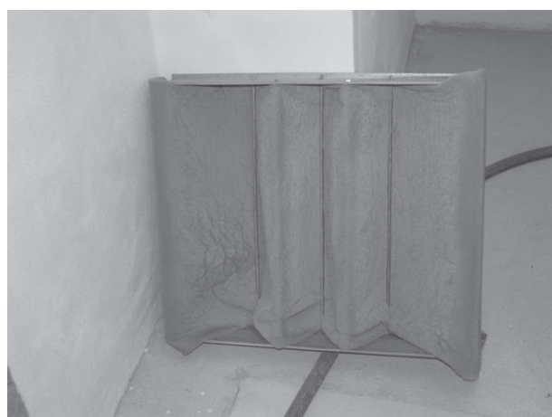
Fig. 3. Polluted filter of outside air filtration
