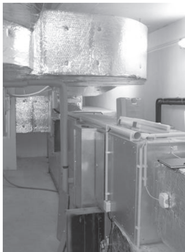
Fig. 2. Chamber with air-conditioning equipment
